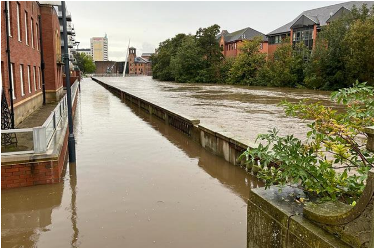
The flood walls by Riverside Chambers kept the river at bay during Storm Babet, 21 October 2023.
